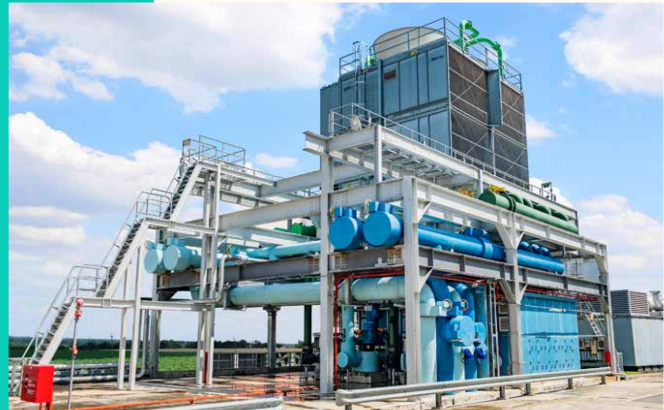
Chillers at PDG's SG1 in Singapore
