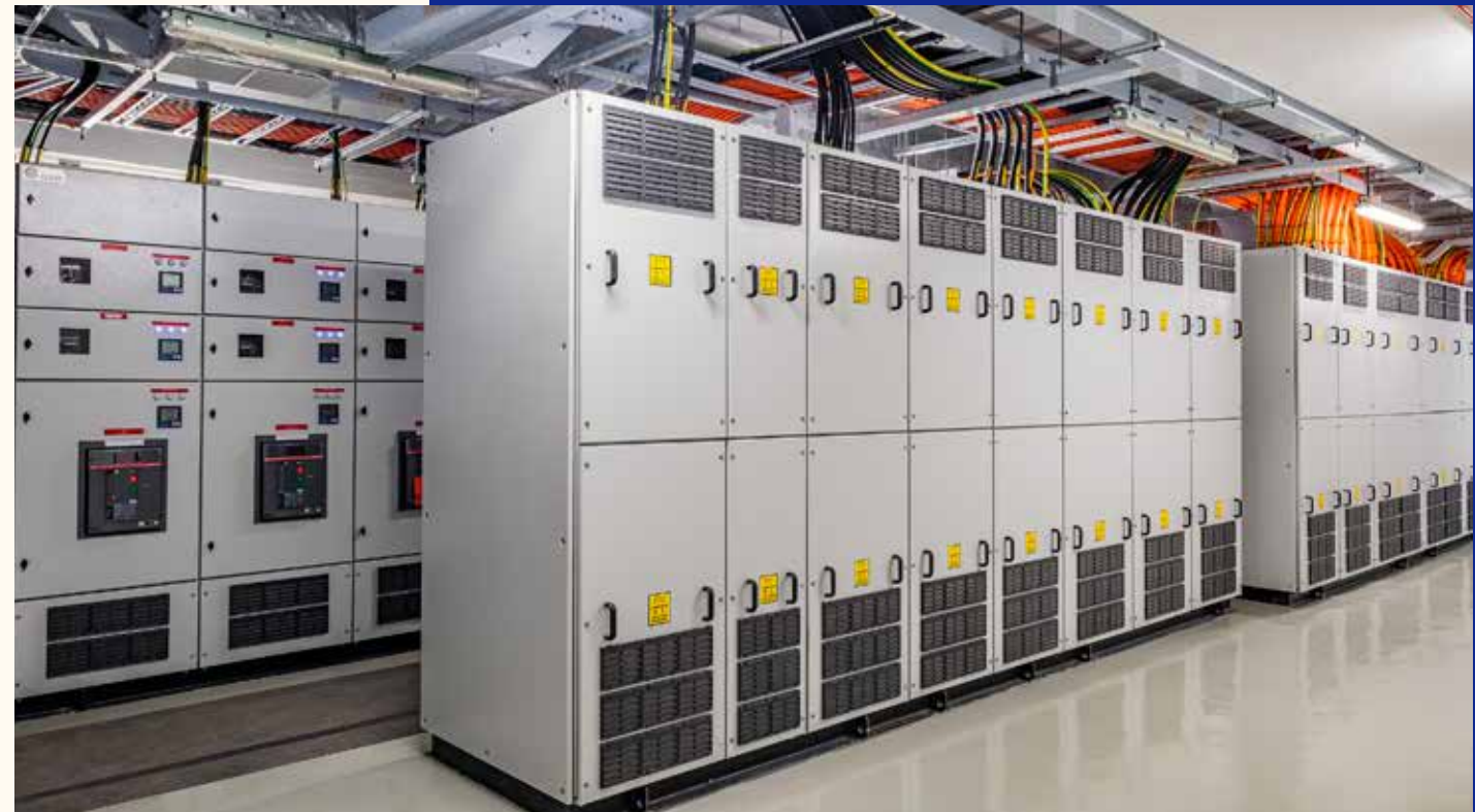
UPS Switchboard at PDG's SGI in Singapore
